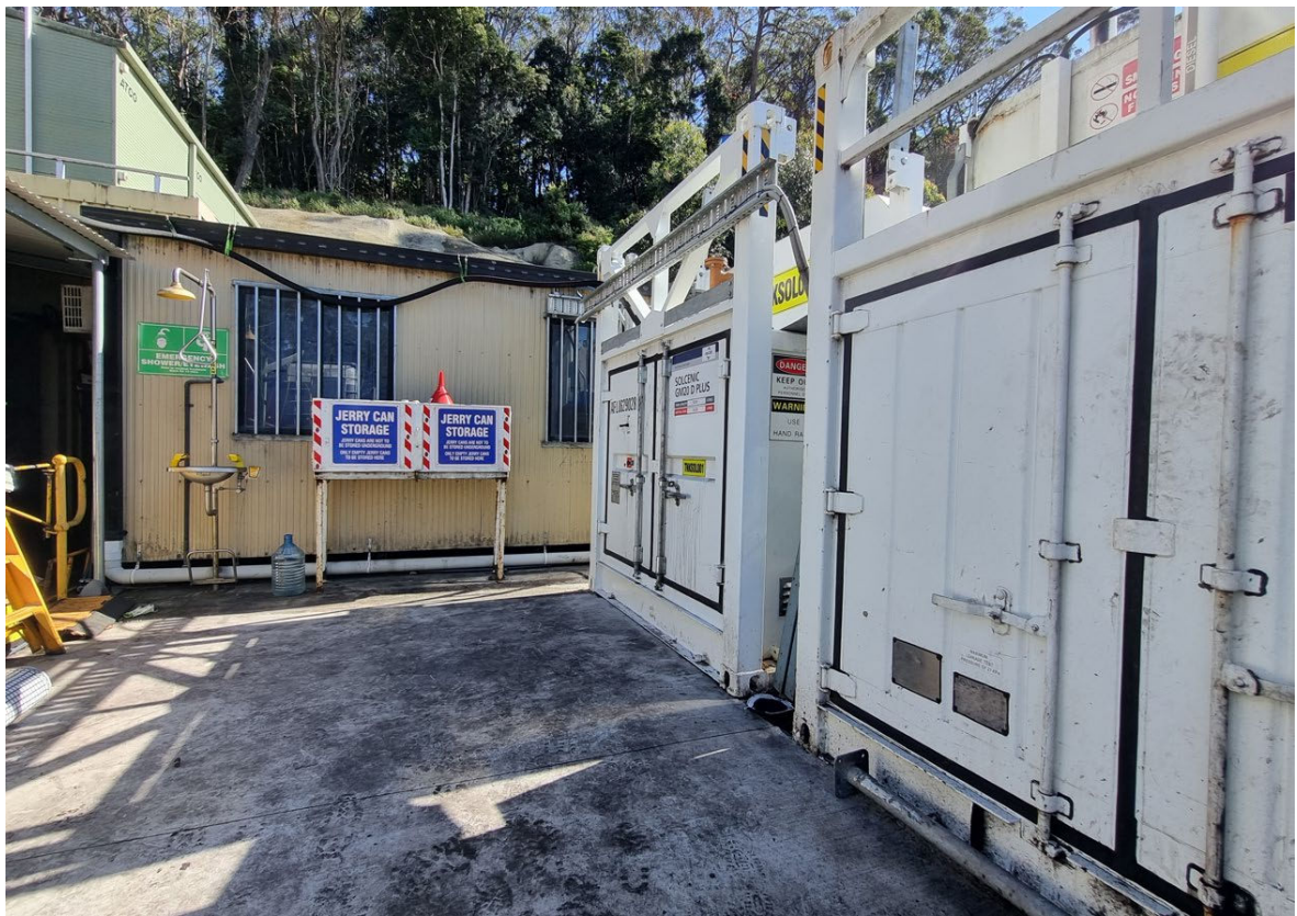
Plate 3: Concrete hard stand around self-bunded diesel and solcenic tanks
